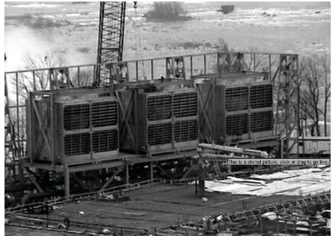
Figure 2. Proximity of cooling towers with the waterfalls (located near the left side of this picture taken during construction).
