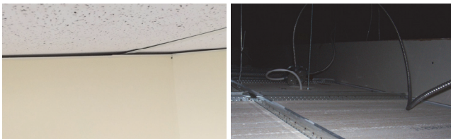
Figure 1: Demising wall shown to extend only to the underside of the ceiling (left), and slightly above the ceiling (right).
