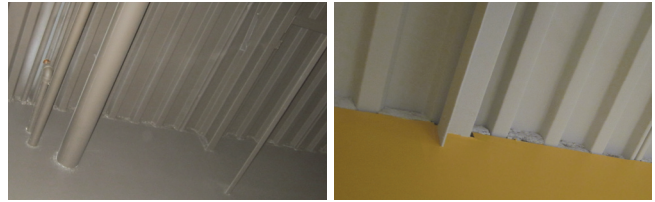
Figure 2: Junction between demising wall and ceiling deck, and penetrations shown sealed (left), and filled but not sealed (right).
