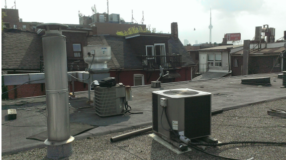
Figure 1: Roof top noise impacting nearby balcony in Toronto.
