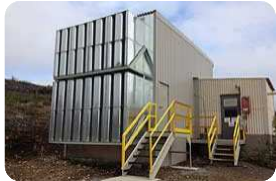
Figure 4: Ventilation system after control
