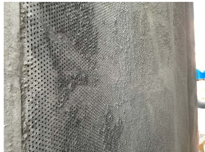
Figure 2: Clogged Perforations in Baffle Casing
