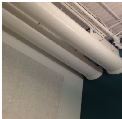
Figure 2: Supply Air Ducts passing between Band Room and Dance Studio.
