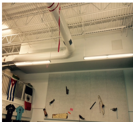
Figure 3: Bulkhead Around Supply Air Ducts in Band Room.
