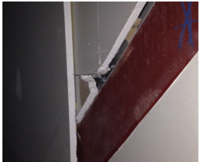
Figure 1: Bridging of Theatre/Atrium wall cavity by structural steel cross bracing.
