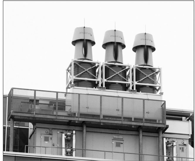
Figure 2: Noise Abatement Measures Installed on an Air Induction Exhaust Fan System
