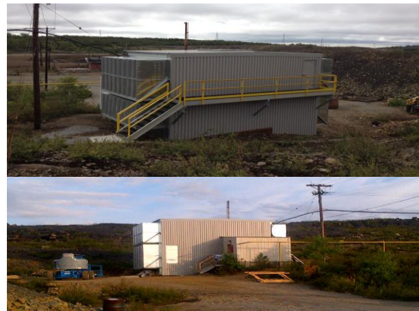
Figure 2: After the ventilation system
