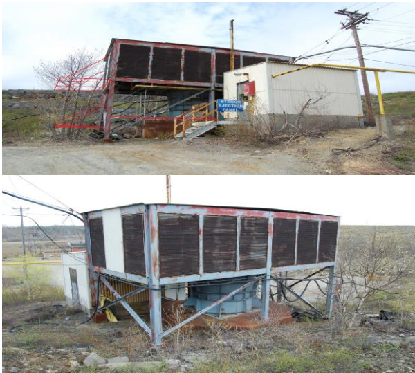
Figure 1: Before the ventilation system
