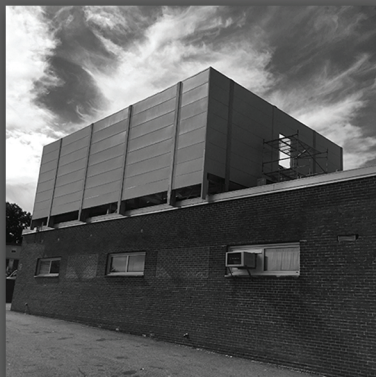
ROOFTOP NOISE BARRIER WALL SYSTEM
