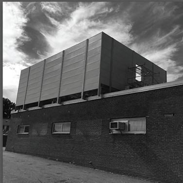
ROOFTOP NOISE BARRIER WALL SYSTEM
