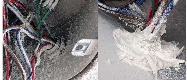
Figure 1: Unsealed Conduit Opening in Fire Alarm Junction Box (Left), and Conduit Opening after Applying Sealant (Right)
