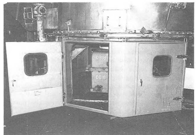
Photo 2. Front Closure Panel - Gearbox visible through door.
