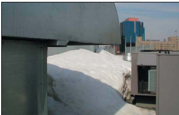
Figure 1: Photo of Snow Accumulation on Roof
