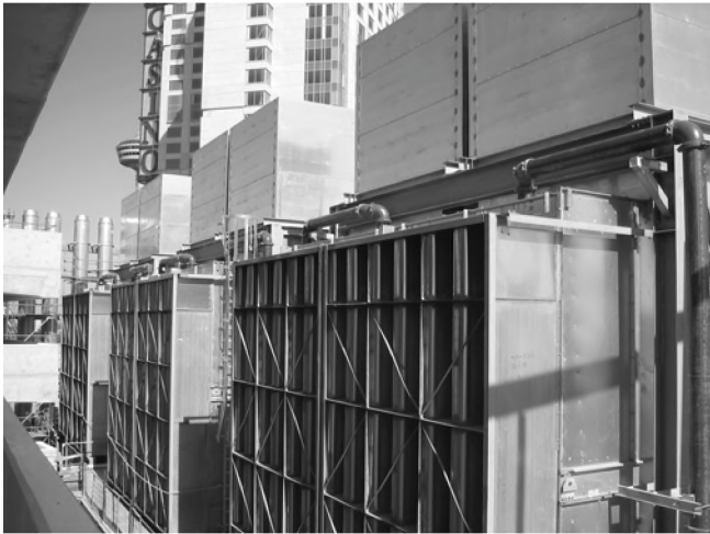
Figure 3. Installed discharge and intake silencers.
