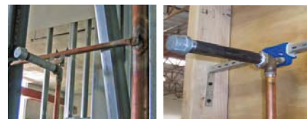
Fig 1.3 Shower head support compared to an engineered anchor point
