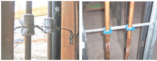
Fig 1.4 Mid-span support (vertical/horizontal) showing a questionable use of felt and tie wire, and to engineered tube clamps
