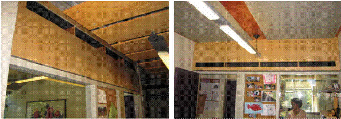
Figure 10: Drawing and photographs of the lined, Z-shaped silencer installed in the Liu office-partition opening.
