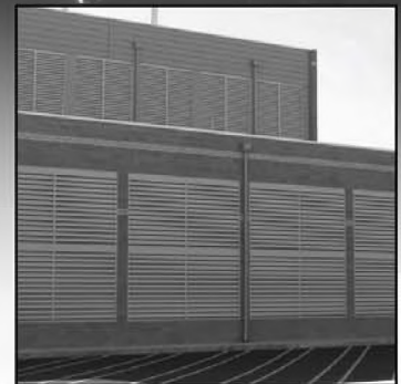
Central Energy Plant Louvers
