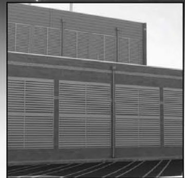
Central Energy Plant Louvers
