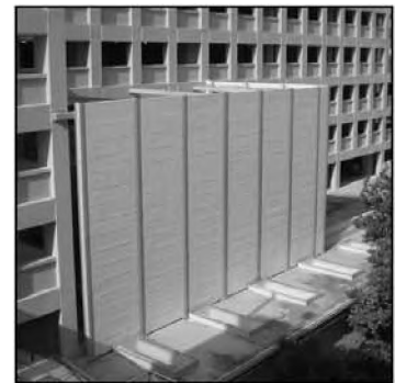
Cooling Tower Barrier Wall System
