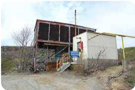
Figure 3: Ventilation system before control
