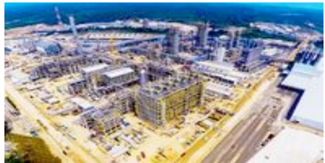
Figure 1. Braskem-Idesa, Etileno XXI Facility, Coatzacoalcos, Mexico
