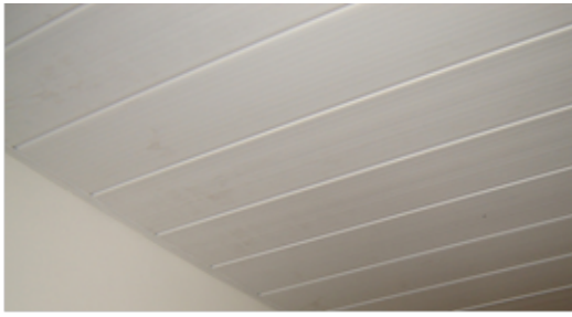
Figure 2: PVC ceiling panels.
