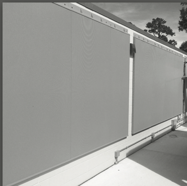
EQUIPMENT YARD NOISE RIGID ABSORPTION PANELS
